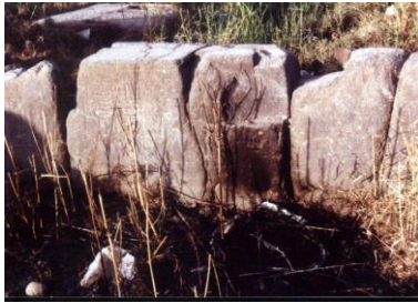
Fig. (1): Basaltic blocks highly cracked due to weathering & plant vegetation, Memphite
