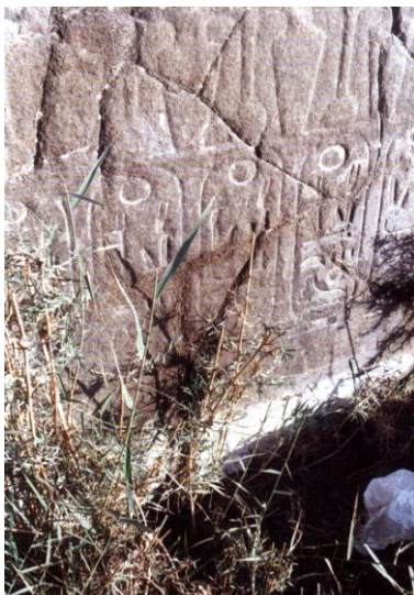
Fig. (5): Basaltic block showing white salt efflorescence at its base & coarse single cracks, Memphite.
