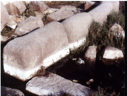
Fig. (3): Field view showing parts of basaltic blocks immersed in domestic water. Salt efflorescence can be noted
